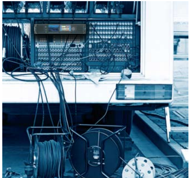
PHABRIX Rx 2000 in the tail gate of an OB truck - feeds via HDMI/SDI to the control room inside the truck.
