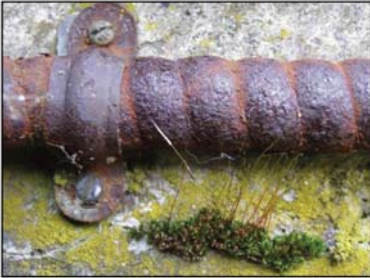
Figure 30. Cleaning up sources of PIM can cure interference problems
