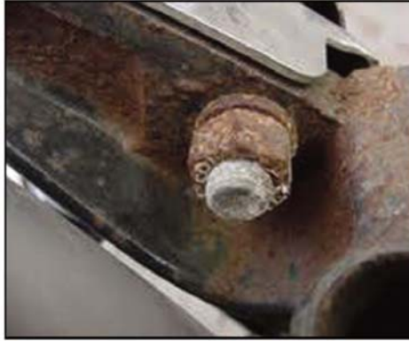
Figure 11. Rusty Bolts can cause PIM.
