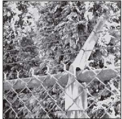
Figure 5: Rust near the transmitter
